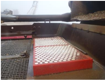
2011 photo of K-Redi-Liner ® Ceramic in place after 6.5 years
